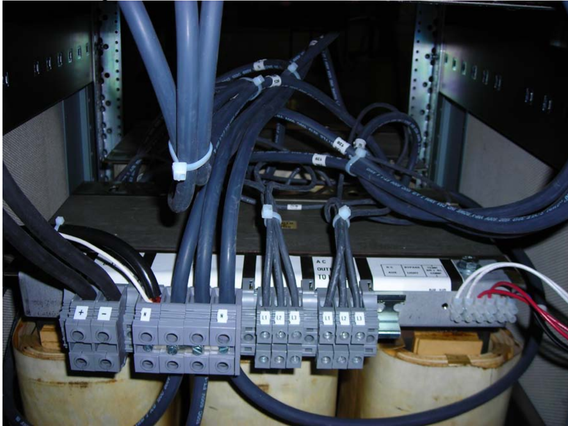
I/O Terminal Block, located at rear of UPS
